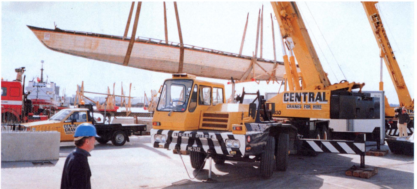
TARATAI coming off the OWENS HEAVY-HAUL truck high above the HOBSON WHARF site about to be settled into place by CENTRAL CRANES.
